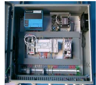
Standard Control Panel with Allen-Bradley PLC and Honeywell Flame Safeguard.
